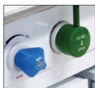
Gas outlet/valve type and location
