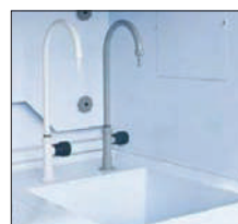
Sink and additional water faucet
